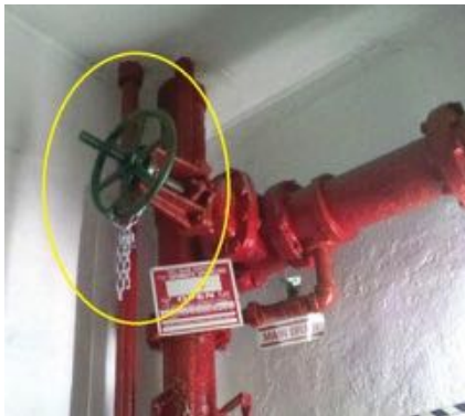
The green valve is a floor control valve. In this photo, the control valve is in the open position.
