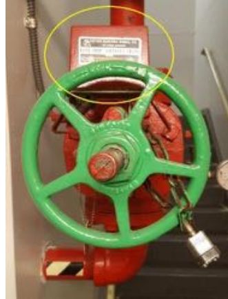
Tamper switch on a sprinkler valve
