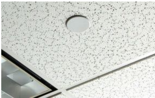
Concealed fire sprinkler heads with cover plates
