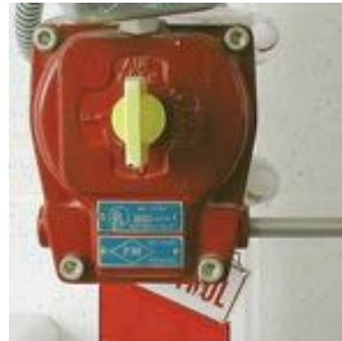
The picture shows the control valve is in the closed position.
