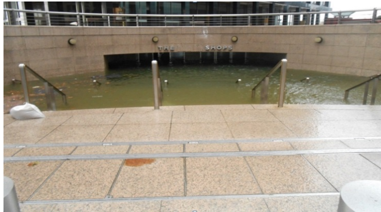
Hurricane Sandy brought the water level up over this shopping premises entrance.
