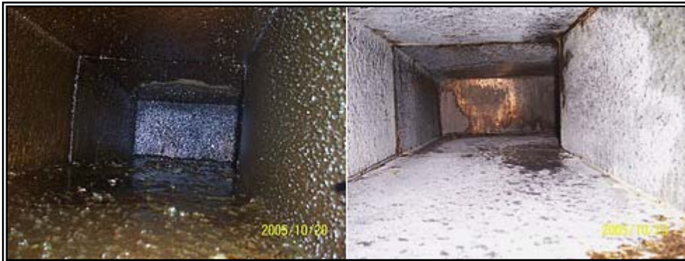
Grease in Duct
